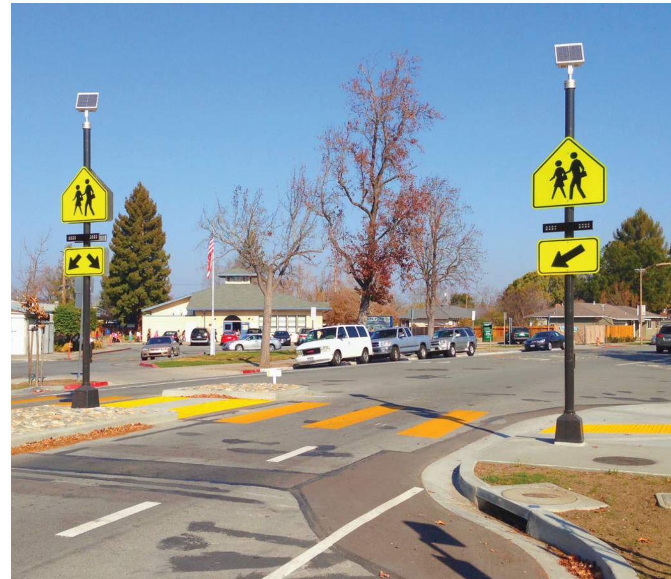
RAPID FLASHING BEACON
